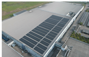
Solar panels on the roof of Factory 1 (Indonesia)
