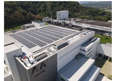
Rooftop solar panels
